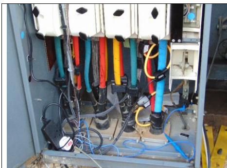
LV Fuse board fitted with GridHound Sensors and Flexible Rogowski Coils.
