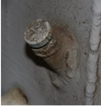
Examples of transformer oil pocket & cap.
